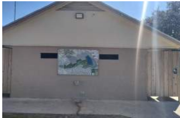
The existing restroom near the baseball/softball complex is aging and due for replacement.
